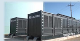
Stationary generator ( '20.10~, demonstration projects, 500kWx2)
